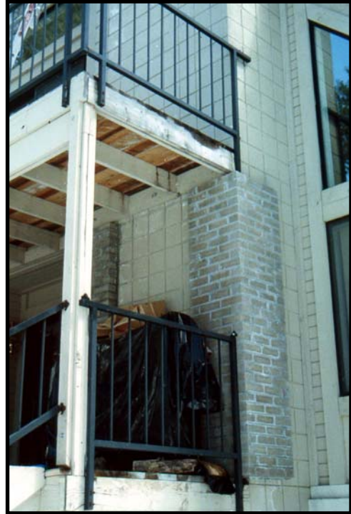
2. Originally the cracks developed in the lower portion, and the contractor "patched" them by covering them with a brick overlay.
