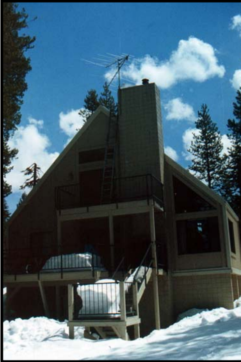
1. This home in Chester developed cracks in the masonry chimney.
