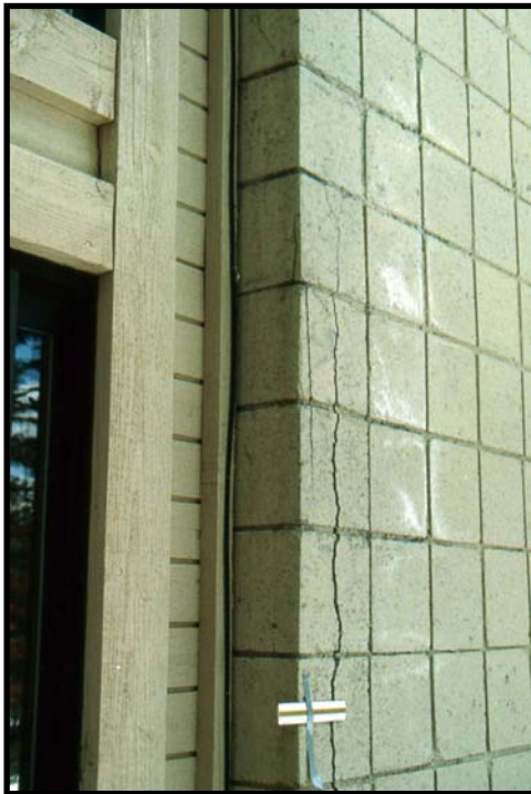
3. Subsequently, cracks also developed in the upper portion.
